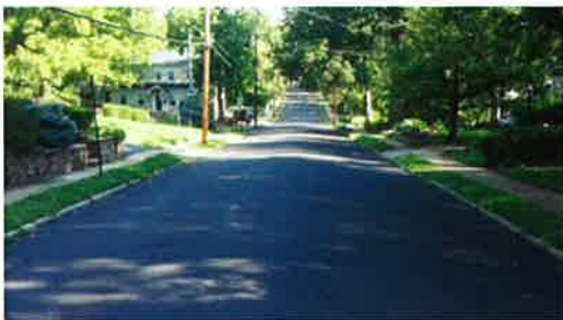
A two year old 1/4" trap rock CHFRS2P chip seal system in Webster Groves is performing well.
