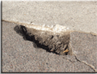
Clear pothole of loose debris and pour HP into the hole or utility cut.
