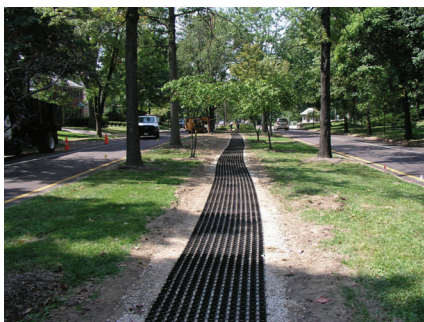
Grasspave2 was installed over a prepared sub-grade with a drainable aggregate base.
