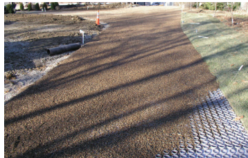
A GravelPave 2 project nearing completion. Once the grids are full, service driveway will be constructed.
