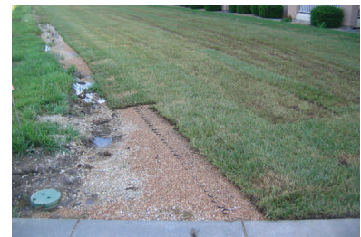
A Grasspave 2 system forms an extension to the paved parking adjacent to an apartment complex.
