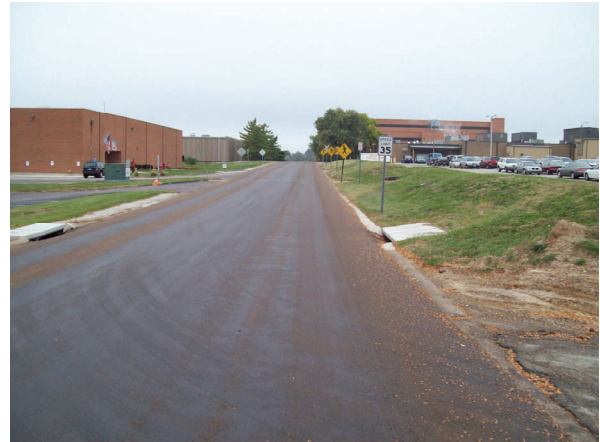
This street had a skid number of 25 after a pavement rejuvenator application. The mini-mum safety threshold value for low volume roads is 30.
