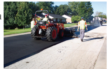
The paving fabric is applied in the first phase of the operation.
