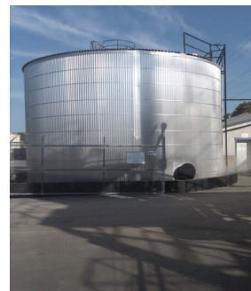
This 80,000 gallon emulsion tank at Bi-State Emulsions contains a steam coil heating system and a propeller style agitator.
