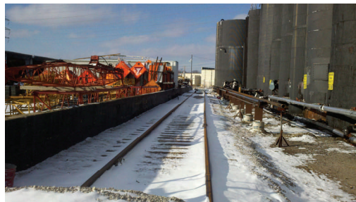
A new rail system was installed along the western perimeter of Missouri Petroleum’s yard
